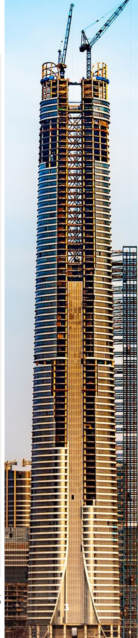
Right: The Iconic Tower under construction in the New Administrative Capital (NAC), March 2022. Credit: Youssef Abdelwahab/Unsplash
