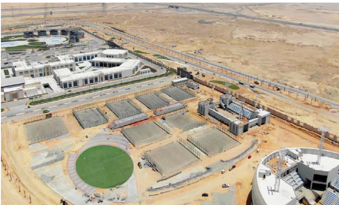
The Egyptian regime hopes to host the 2036 Summer Olympics in the NAC's Olympic City, shown under construction in the above undated photo. Photo: Concord for Engineering and Contracting
