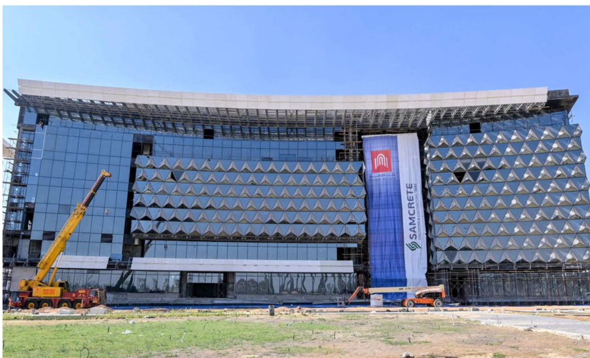
Samcrete Engineers and Contractors, a subsidiary of Samcrete Holding, constructs the Banque du Caire headquarters, pictured above in an undated photo, in the NAC. Photo: Samcrete Engineers and Contractors
