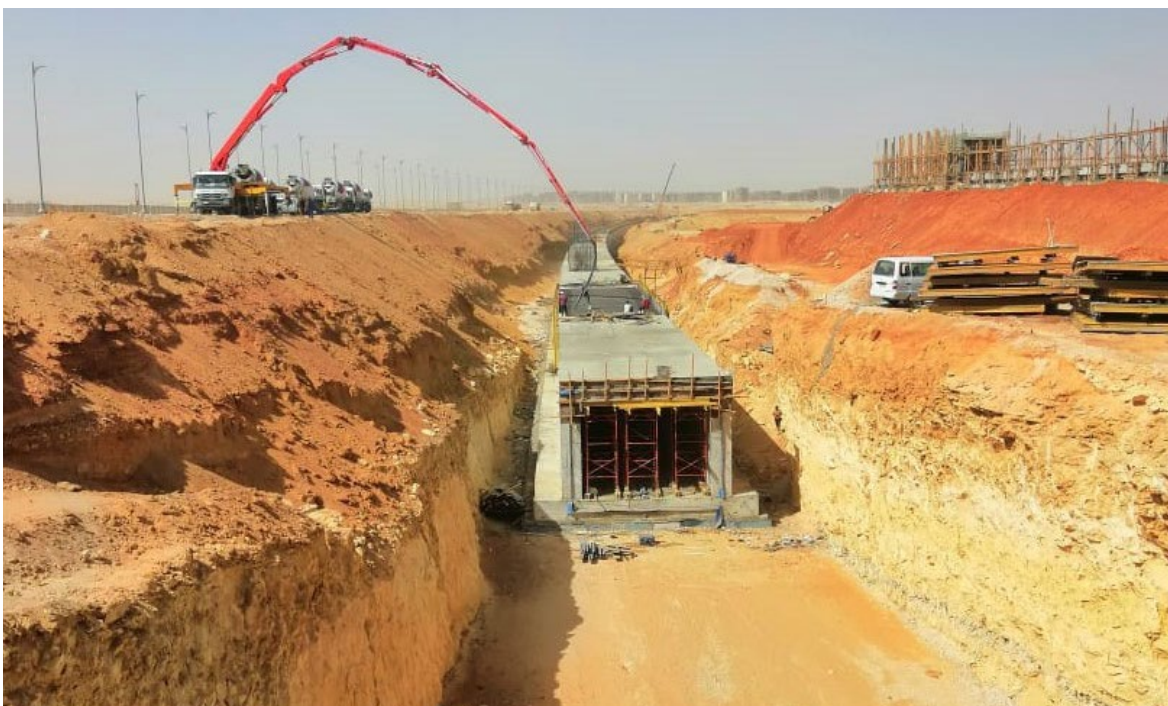
Concord for Engineering and Contracting constructs a utility tunnel in the NAC in this undated photo. Photo: Concord for Engineering and Contracting
